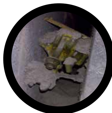
Spot the scaffolding clamp!
