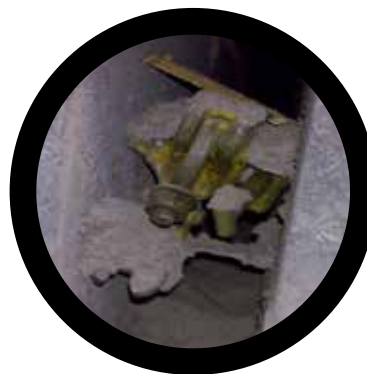
Spot the scaffolding clamp!
