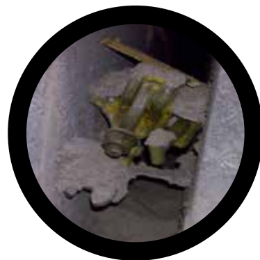
Spot the scaffolding clamp!
