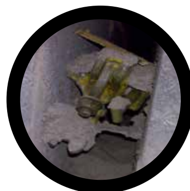
Spot the scaffolding clamp!
