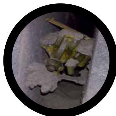
Spot the scaffolding clamp!
