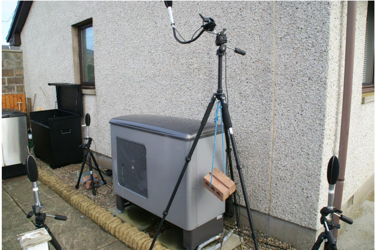
Picture 5-14. 422 Fraserburgh, Replacement ASHP and Microphone Arrangement
