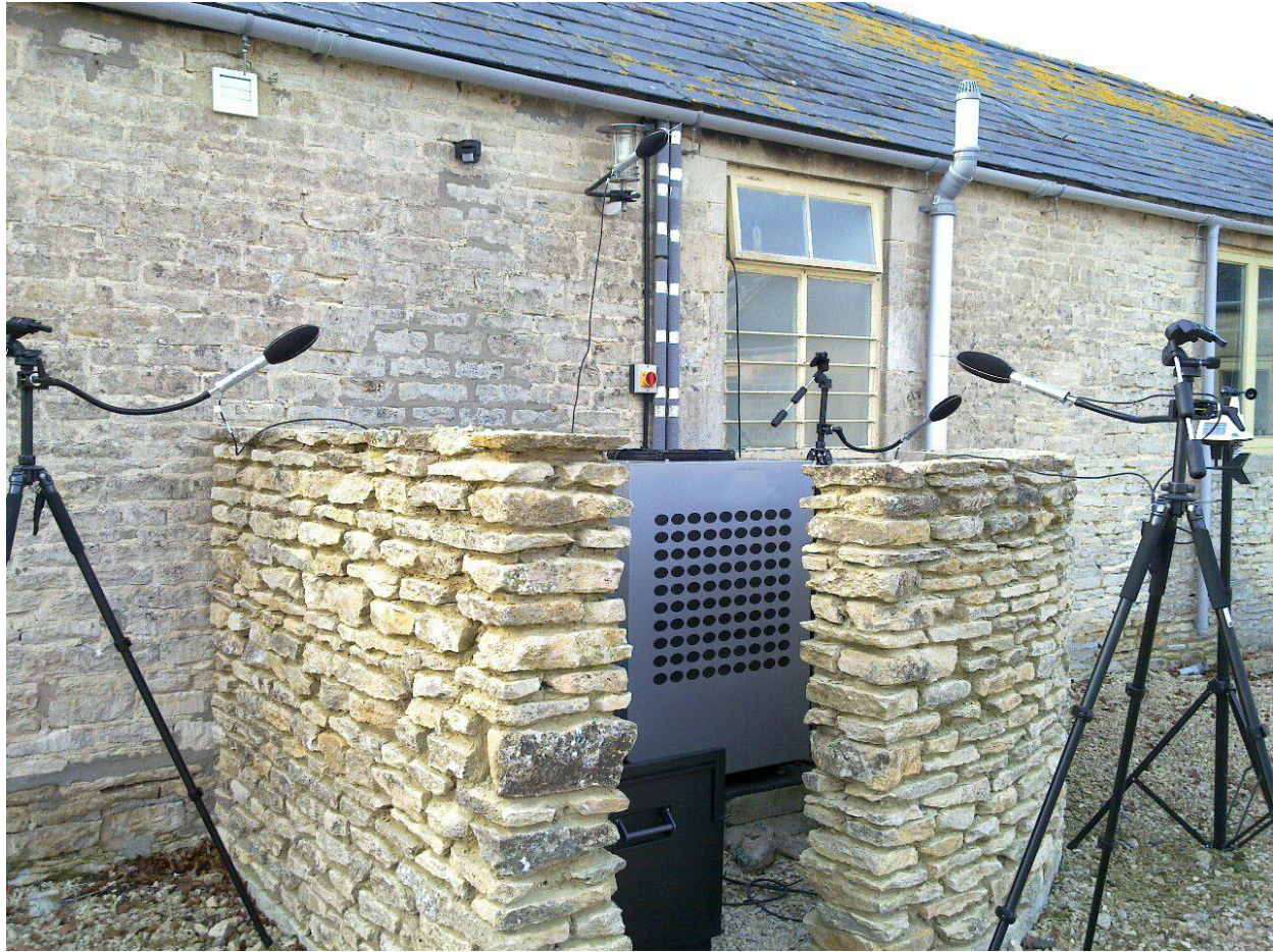
Picture 5-23. 478 Cotswold (Courtyard), ASHP and Microphone Arrangement
