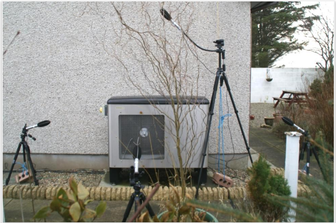
Picture 5-12. 422 Fraserburgh, Original ASHP and Microphone Arrangement
