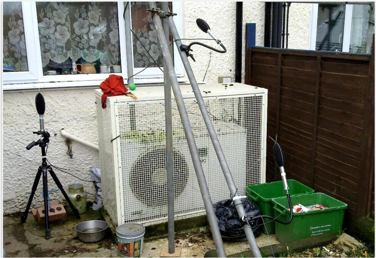
Picture 5-18. 474 West Berkshire (Site 1), ASHP and Microphone Arrangement
