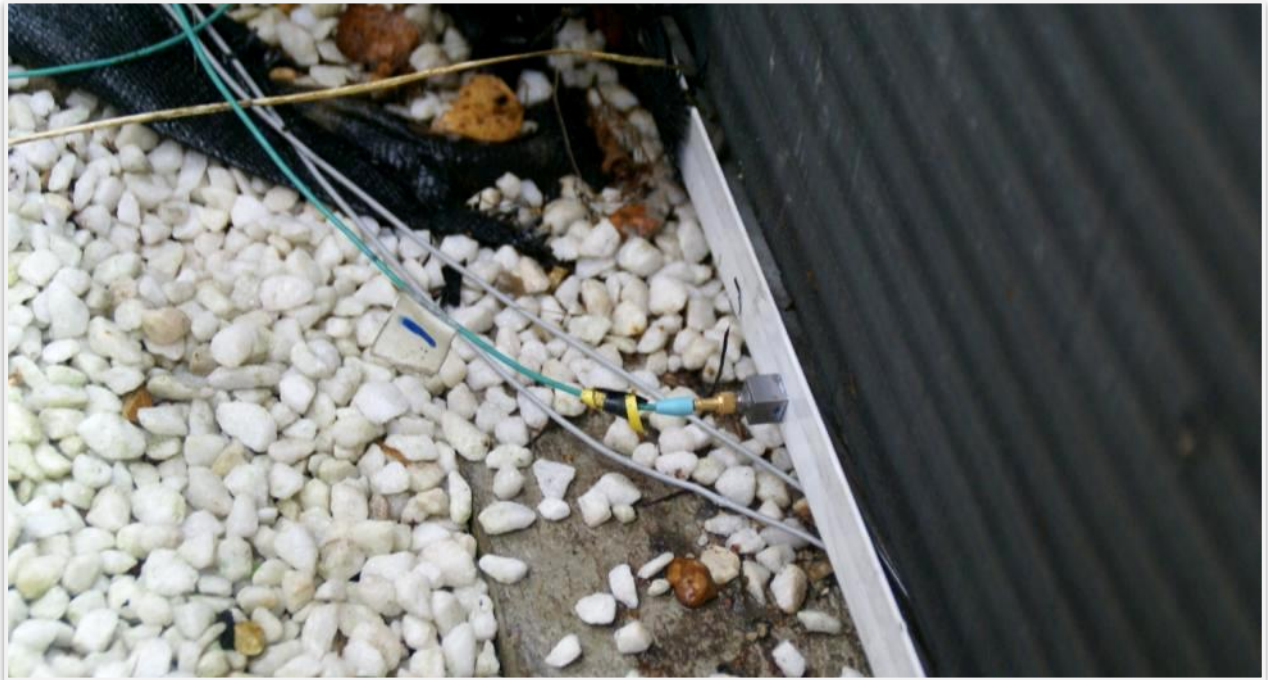
Picture 5-19. 475 West Berkshire (Site 2), Casing-mounted Accelerometer
