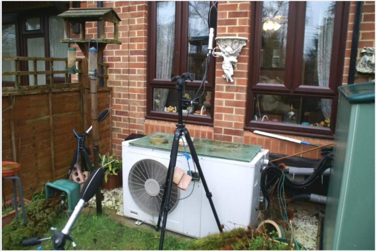
Picture 5-21. 475 West Berkshire (Site 2), ASHP and Microphone Arrangement
