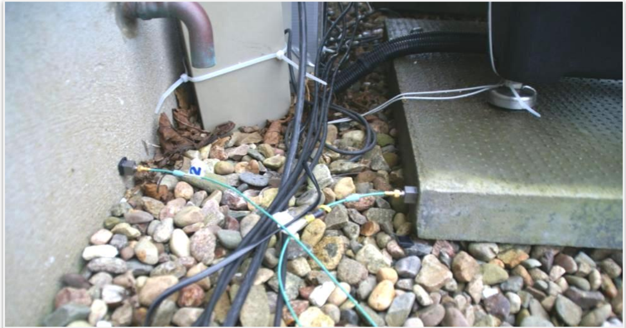
Picture 5-10. 422 Fraserburgh (Original), Footing and Wall-mounted Accelerometers
