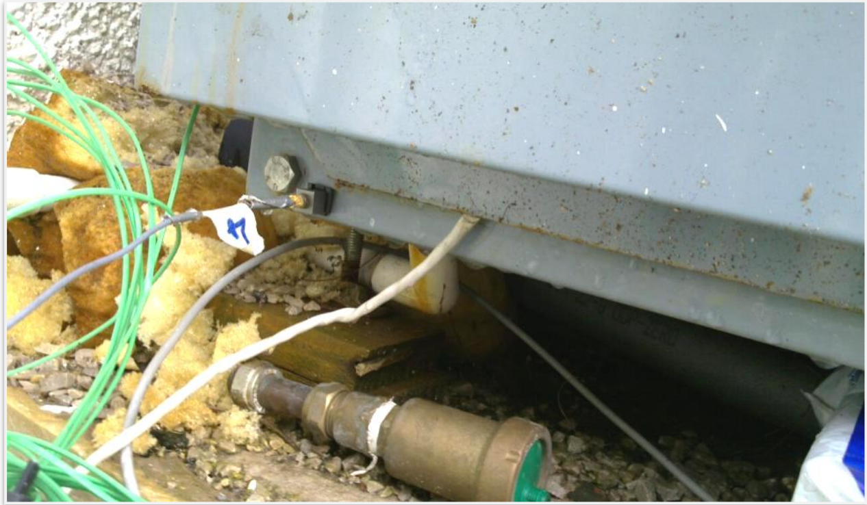
Picture 5-5. 440 Fylde, Casing-mounted Accelerometer
